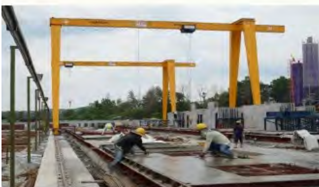
3. After pouring the cement, they need to flatten the surface & let it dry.
