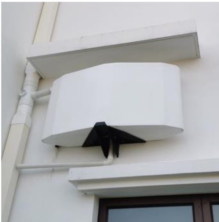
Figure 3: Rainwater Harvesting System
